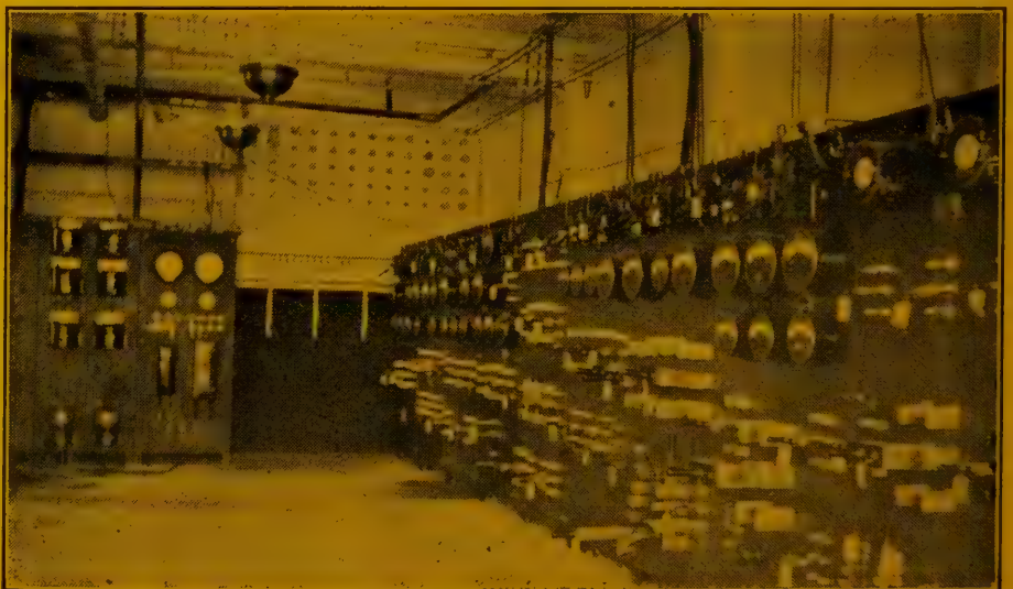
INTERIOR VIEW SHOWING ONE OF OUR HUGE SWITCHBOARDS
